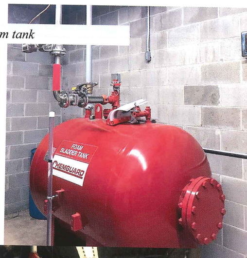
Riser room B
